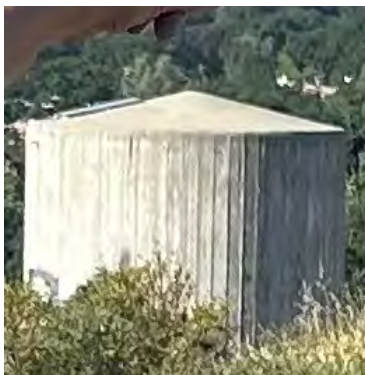
The water tank on LCLT property that will be painted with donated funds.
